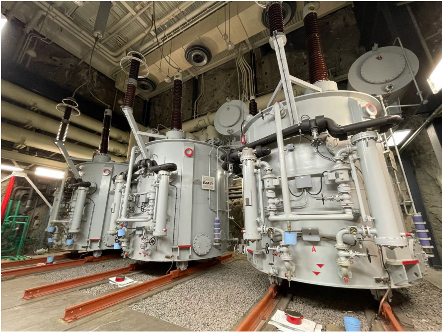
Figure 21: Morrow Point powerplant
