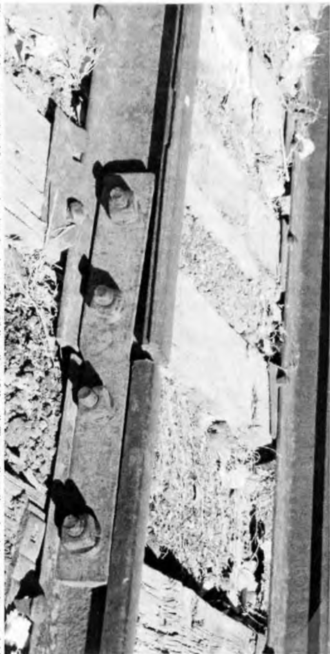
Close up of the wye switch in Montrose showing the change from 90 lb. rail to 65 lb. rail. The smaller rail on the right at one time was laid to narrow gauge width. As you can see the rail joiner had to be cut down to allow the two rails to be bolted together. Photo by Wayne Darling, 24 November 2002.
