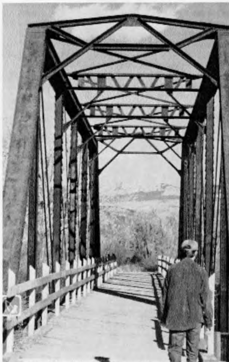
This photograph shows the steel through truss bridge north of Ridgway that is now part of the new bike path. Author included to show scale, 24 November 2002. Photo by Wayne Darling. (Photo courtesy of Matt Darling Collection.)
