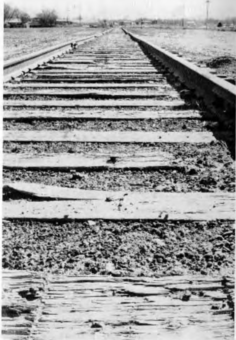
The marks of the old narrow gauge rail can be made out and one of the track spikes missed by the scrapers in 1953 is still in place. The photographer is facing south to Ridgway. Photo by Wayne Darling. (Photo courtesy of Matt Darling Collection.)
