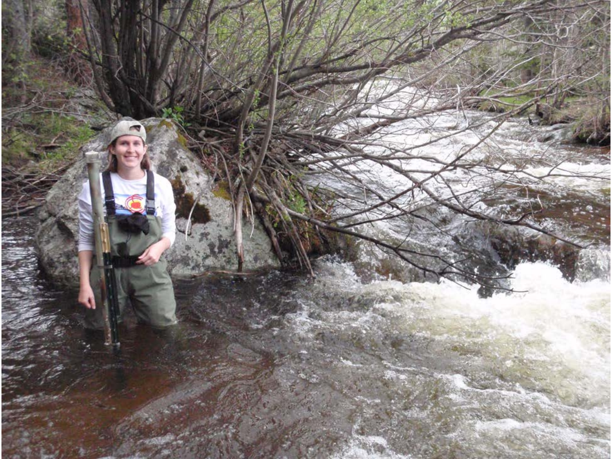
Figure 2. PhD Candidate DeAnna Laurel installing instrumentation to record water height (stage) on Glacier Creek in Rocky Mountain National Park. Photo Credit: Dr. Ellen Wohl.
