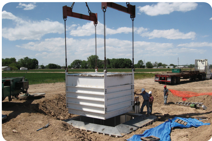
Fig 2: The inner tank plus soil being lowered inside the containment tank. Photo taken by Michael Bartolo.
