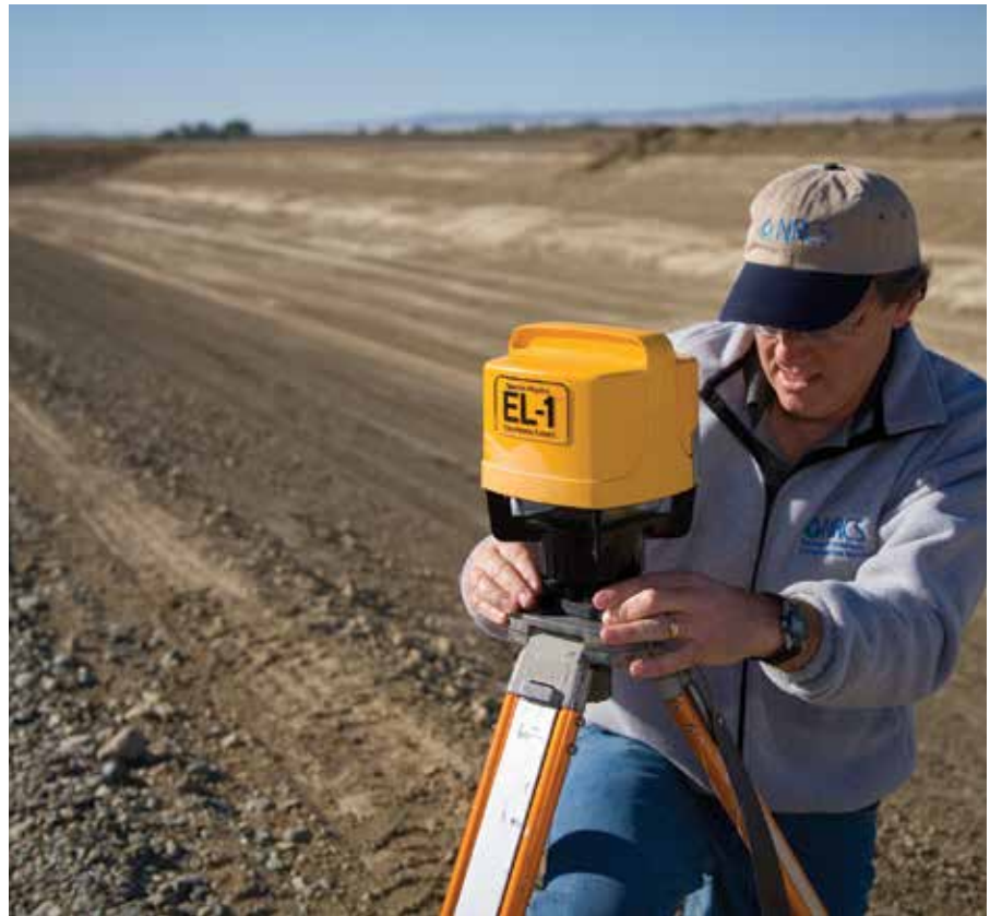
A Natural Resources Conservation Service Area Engineer sets up a laser level to perform a construction inspection on a waste water lagoon for a dairy in Sacramento Valley, California. Photo courtesy of the NRCS.
