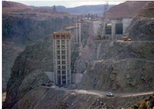
Intake structure for the Blue Mesa Dam, Gunnison River, October 1964 (Ival V. Goslin Collection). Both Ival Goslin and Robert Glover took hundreds of photos of Colorado River structures.
