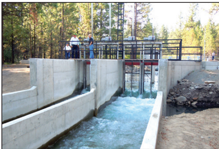
Stakeholders visited a new headgate at the Three Sisters Wychus Creek diversion in Oregon.
