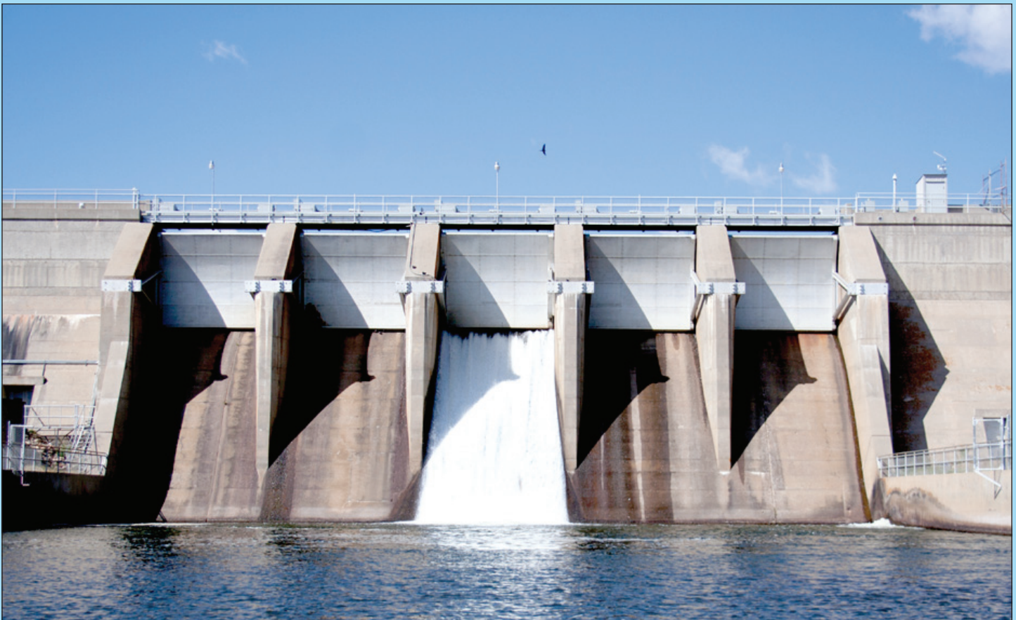
The Estes Powerplant uses Olympus Dam to regulate water levels between Lake Estes and Mary's Lake - water transfer allows the powerplant to generate a small amount of hydroelectricity.
