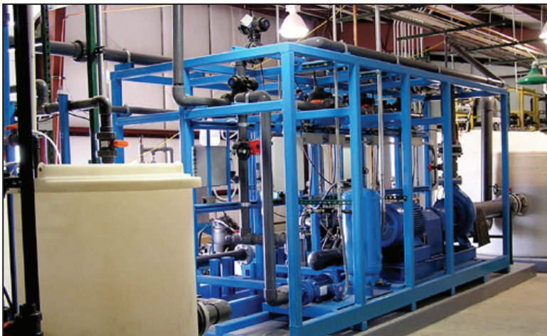
This Stewart Filtration Skid is used for metals filtration and produced water – this is an example of a process that the Colorado Water Innovations Cluster, still in its infancy, might oversee at some point in the future.
