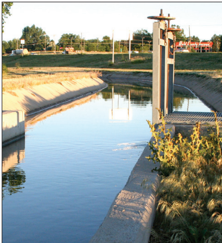
A canal runs along Highway 34 in Greeley, Colo. This water supply will be tapped by many different users.
