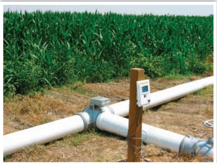
This Hansen displaying logger for WaterMark soil moisture sensors was installed at the top of a corn field near Fowler, Colorado.
