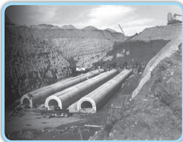
This photo, taken on March 13, 1942, shows the east end of the Alva B. Adams Tunnel during construction.
