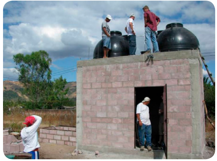
Students and community members installing plumbing to the rooftop tanks for the San Antonio Abad pump house in January 2008
