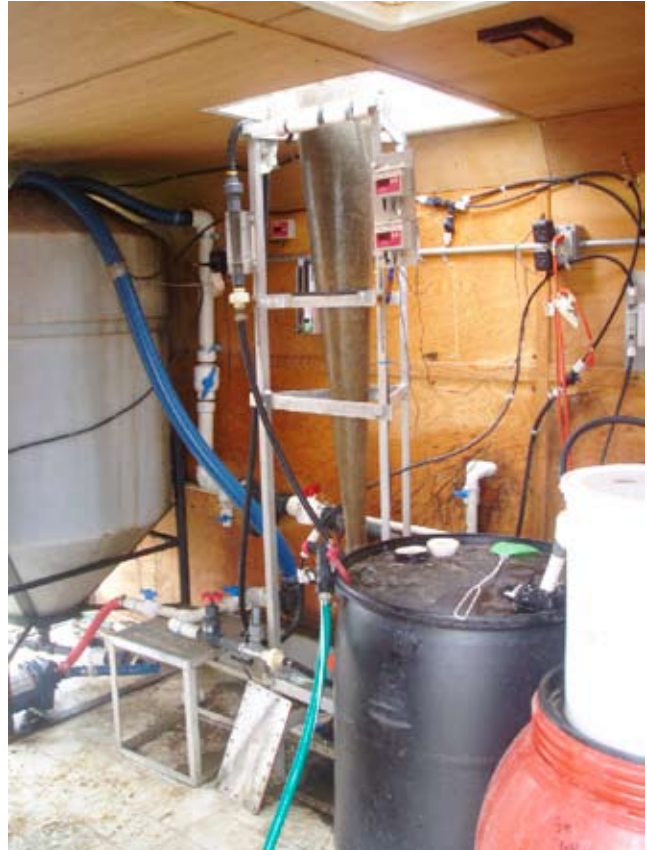
The fluidized-bed reactor was used to treat anaerobic waste lagoon effluent.
