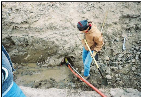
Jet Cleaning of Tile Lines: Modern sewer maintenance technology is very well suited to maintaining buried tile lines throughout the lower valley.
