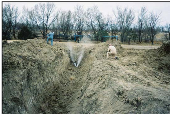
Jet Cleaning of Tile Lines: Photo shows a jet nozzle working through a tile line that has been plugged for many years. The current study estimates that there are approximately 140 miles of old tile lines in the lower Arkansas Valley that need maintenance work of this nature.
