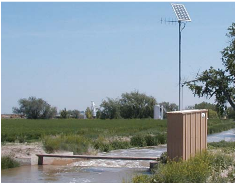
This rated canal section is remotely monitored using a SCADA system. RTU equipment is 12-volt DC powered from a solar panel that maintains a charge on a battery. Communication with the site is by radio.
