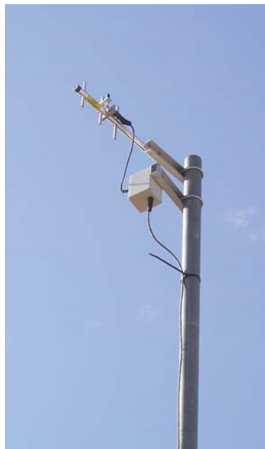
This SCADA system uses spread spectrum radio which does not require federal licensing. The spread spectrum radio is housed in the white enclosure and the directional antenna shown has a line-of-sight range of approximately 5 miles.
