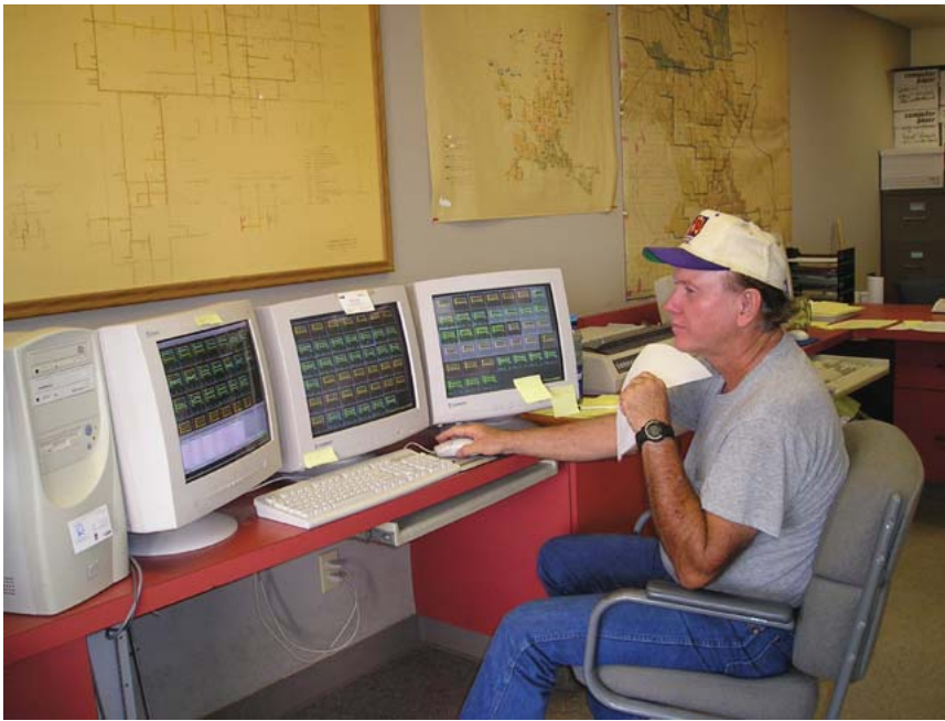
An operator at CAIDD near Phoenix monitors primary flows and water surface elevations in the 60-mile canal. This SCADA system was implemented at relatively low cost using affordable RTU equipment and spread spectrum radios for communication.
