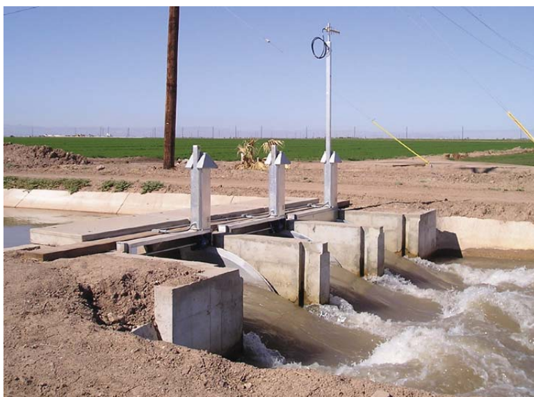
This check structure is controlled by Rubicon gates which are integrated with the SCADA system and used for water surface level control or flow control.
