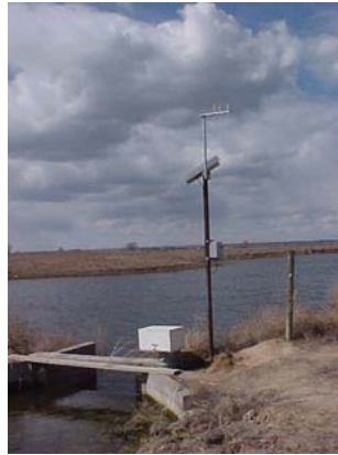
Monitoring and control devices using radio communication such as this one are becoming more affordable.
