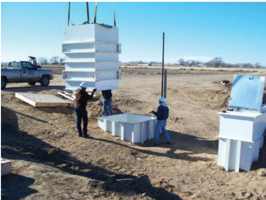
The inner tank with soil being lowered into the containment tank of the lysimeter. The manhole for accessing the underground weighing scale is on the right.
