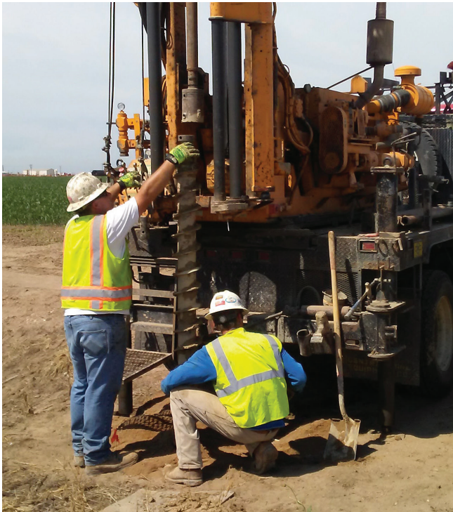
Installation of Groundwater Monitoring Wells in the Gilcrest area, performed by Drilling Engineers, Inc.
