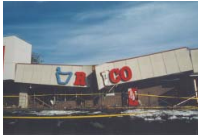
Drug store roof collapsed under weight of snow from March 13, 1993 record snowstorm. Photo by Grant Goodge.
