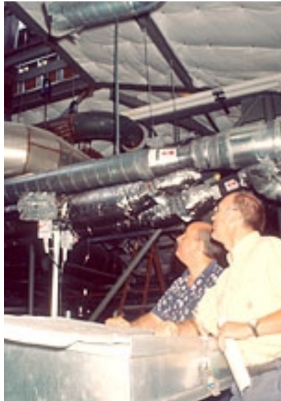
Dr. Steven Higgs and Dr. Allan Roberts check out the air exchange system in the new BioEnvironmental Sciences Building.
