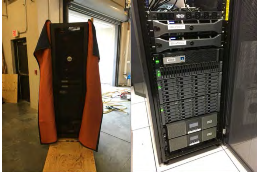
Figure 1. Rack of equipment deployed to the ATCSCC.
