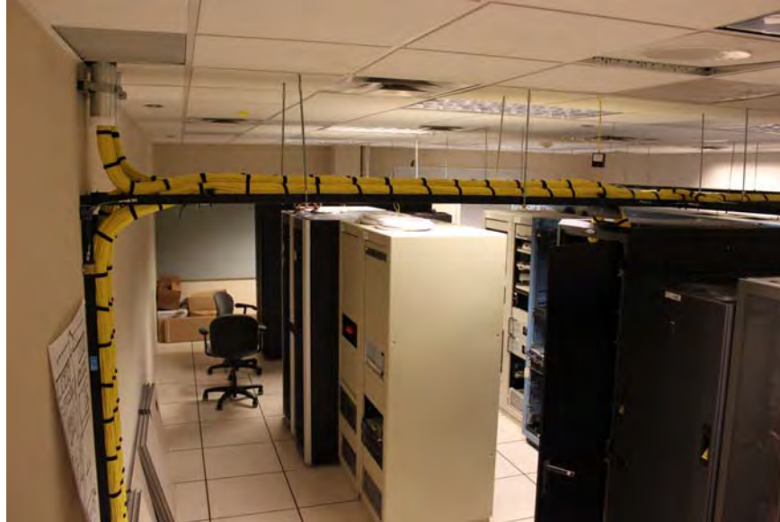
Figure 6. New cabling infrastructure at AWC.
