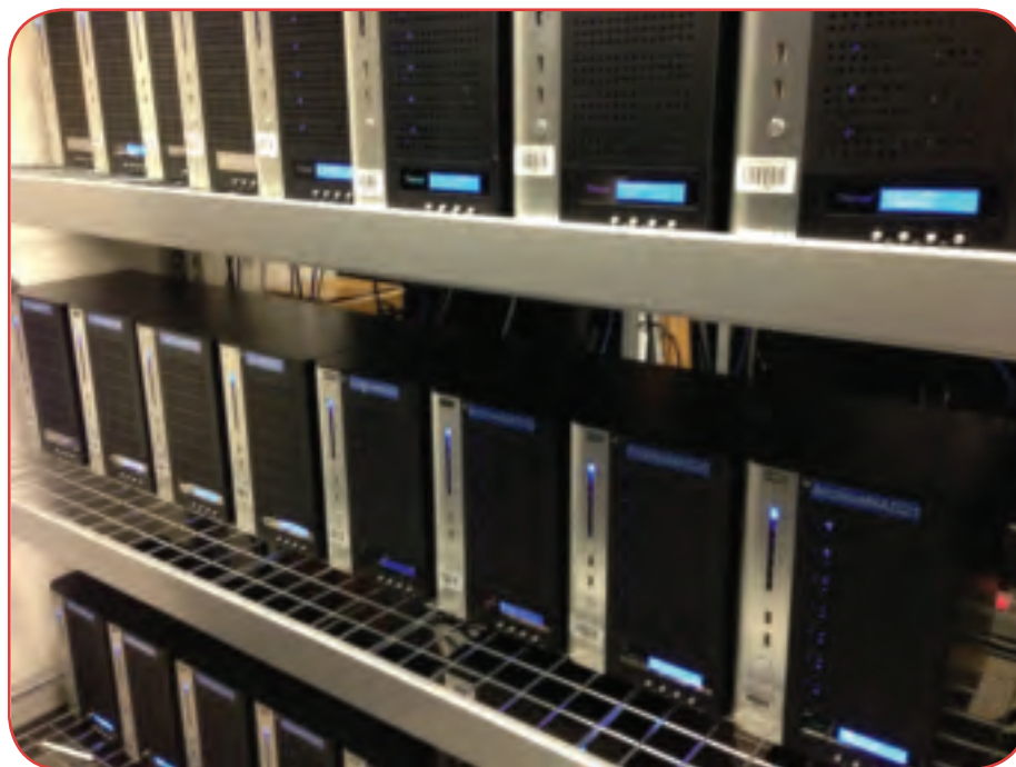
NAS Data Storage Units
