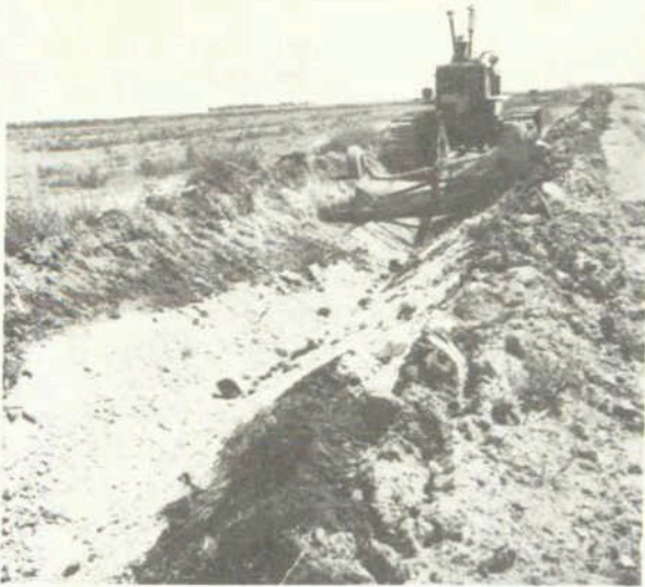
Photo 6--In several instances, the dams of bentonite have been spaced along a canal and then spread with a V-ditcher rather than with water.
