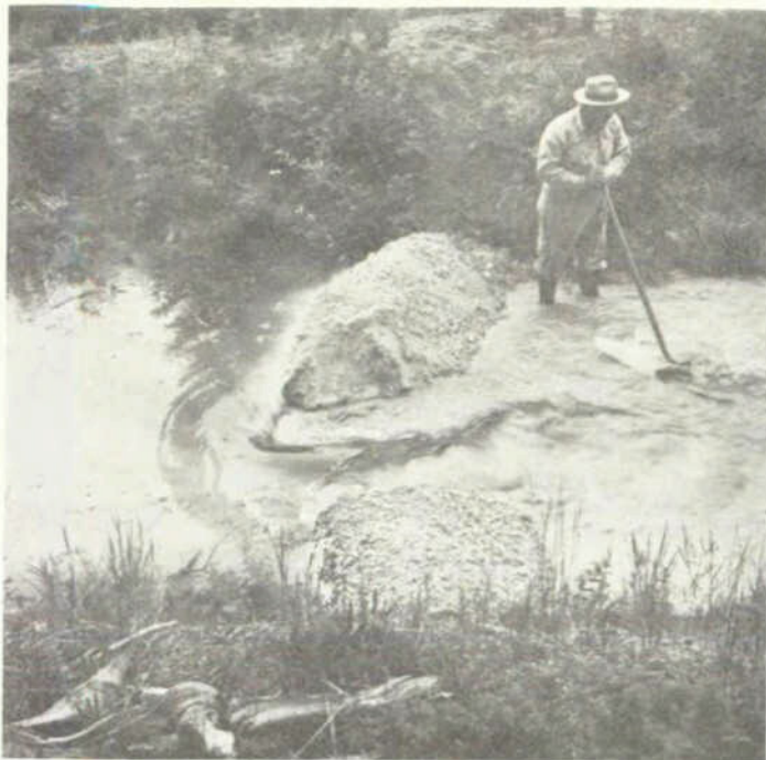
Photo 3--Most common method of application consists of placing dams of bentonite in dry canal, then running in small head of water and washing bentonite down canal.
