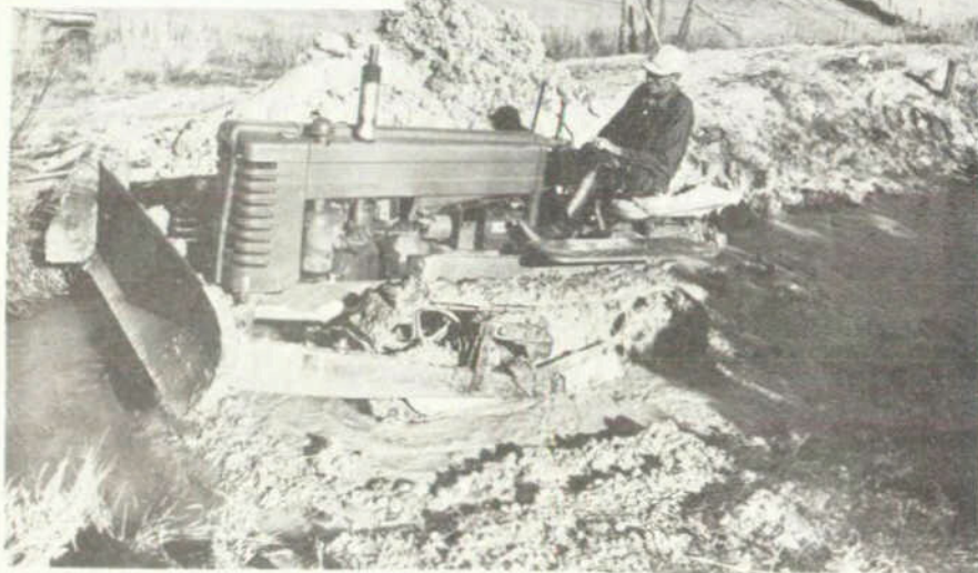
Photo 4--The bentonite can be shovelled into the water as the dam is washed out, but in some cases, as above, a small bulldozer has been used.
