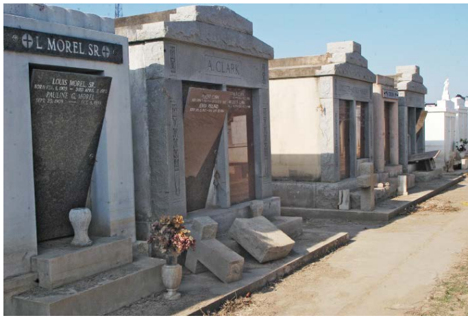
Fig. 10 – Earthquakes fracture and topple stones, and compromise or damage public and family mausoleums © FEMA.
