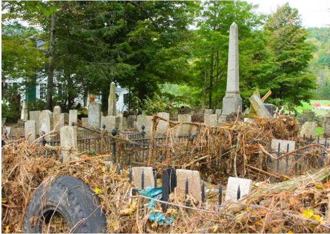
Fig. 4 – Upon closer examination, and after the waters recede, the magnitude of the cleanup that awaits becomes obvious. © FEMA.
