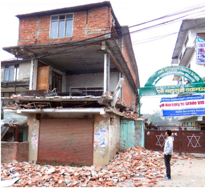
Over 8,000 school buildings were damaged in the earthquake. Here, a young man stares at school desks crushed by soft story collapse. As bricks fall out of unreinforced infill walls, seismic load is concentrated to that floor, causing collapse. @ Anne Sanquini
