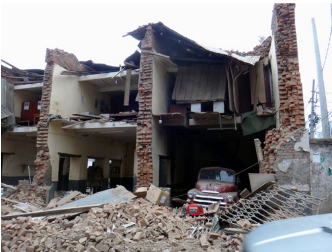
Unreinforced masonry building in foreground collapsed to a pile of bricks while the building in the background is perfectly fine. @ Anne Sanquini
