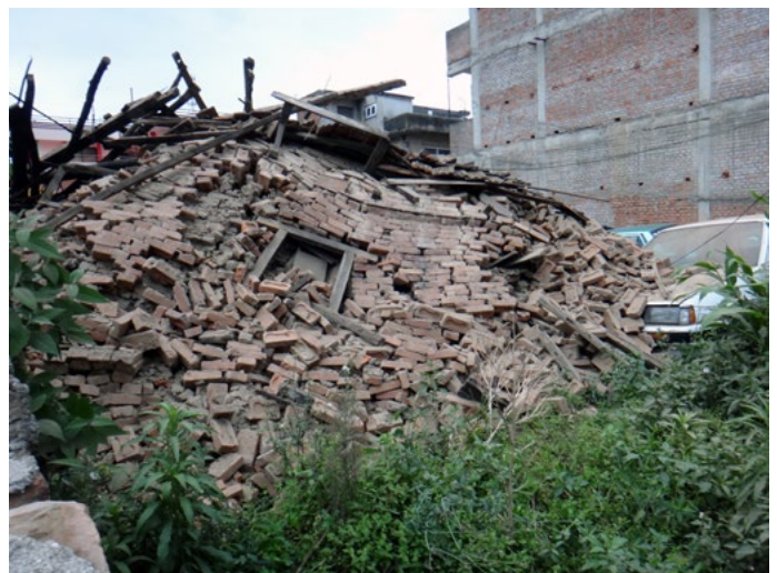
Collapsed unreinforced masonry brick firehouse. @ Anne Sanquini
