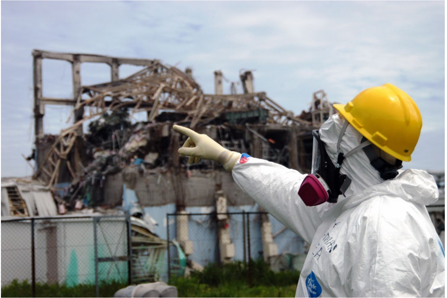
International Atomic Energy Agency fact-finding team leader Mike Weightman examines Reactor Unit 3 at the Fukushima Daiichi Nuclear Power Plant on 27 May 2011 to assess tsunami damage and study nuclear safety lessons that could be learned from the accident. @ IAEA Imagebank Greg Webb/IAEA
