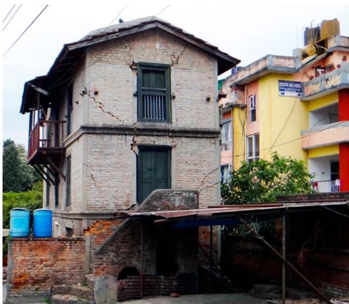
Large cracks have formed in the old, unreinforced masonry building on the left while the newer buildings on the right appear have no visible damage. @ Anne Sanquini
