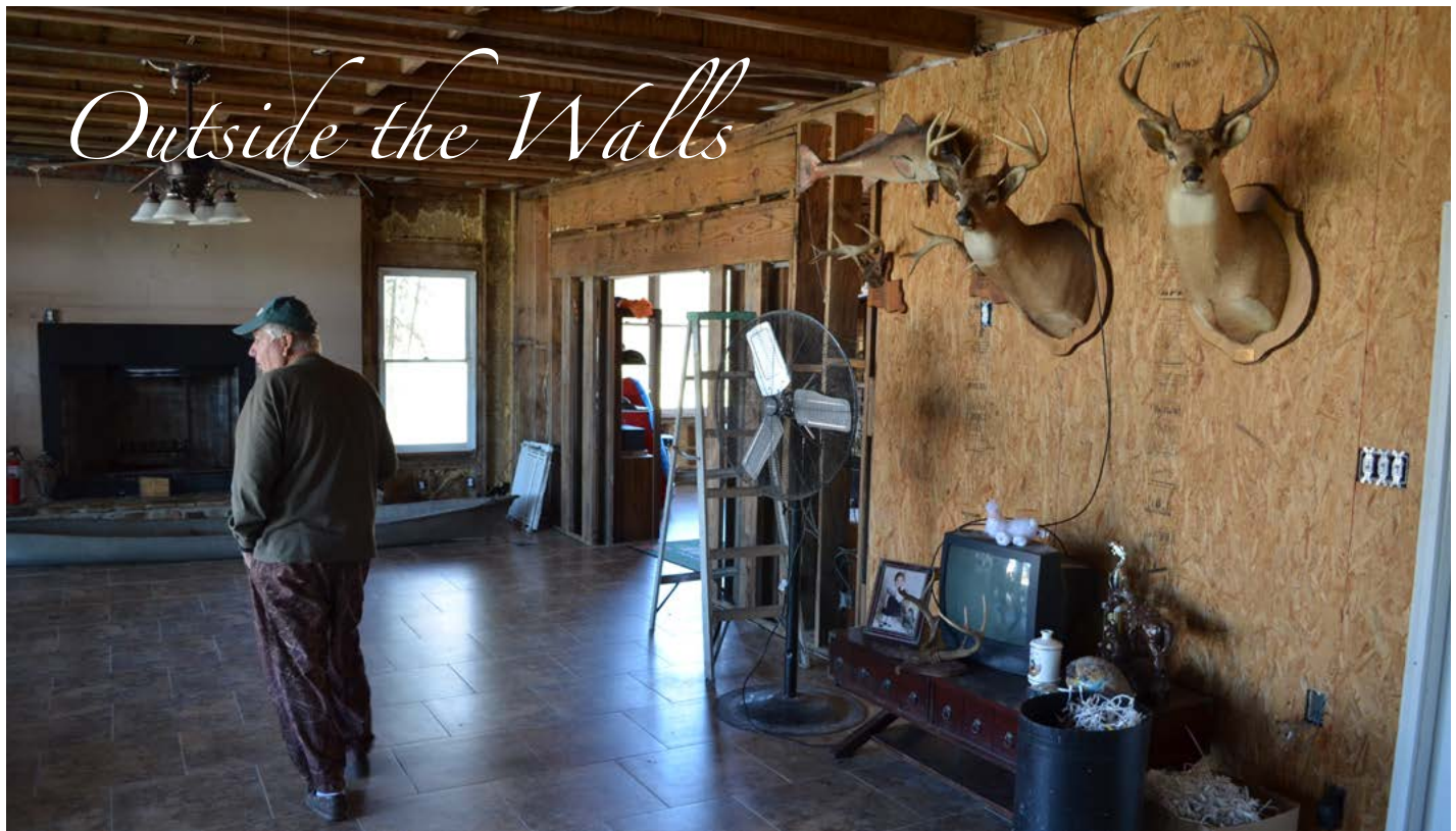
A resident of Braithwaite in the now-abandoned ground floor of his home. Following repeated flooding in Hurricane Katrina and Isaac, the resident moved all of the home's essential functions to the upper floors and now uses the ground floor exclusively for storage. © Zachary Lamb
