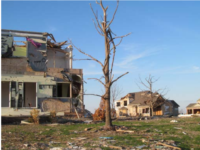
Many of Washington's homes were devastated beyond repair after the November 2013 EF-4 tornado. © Rozdilsky (04/15/14).
