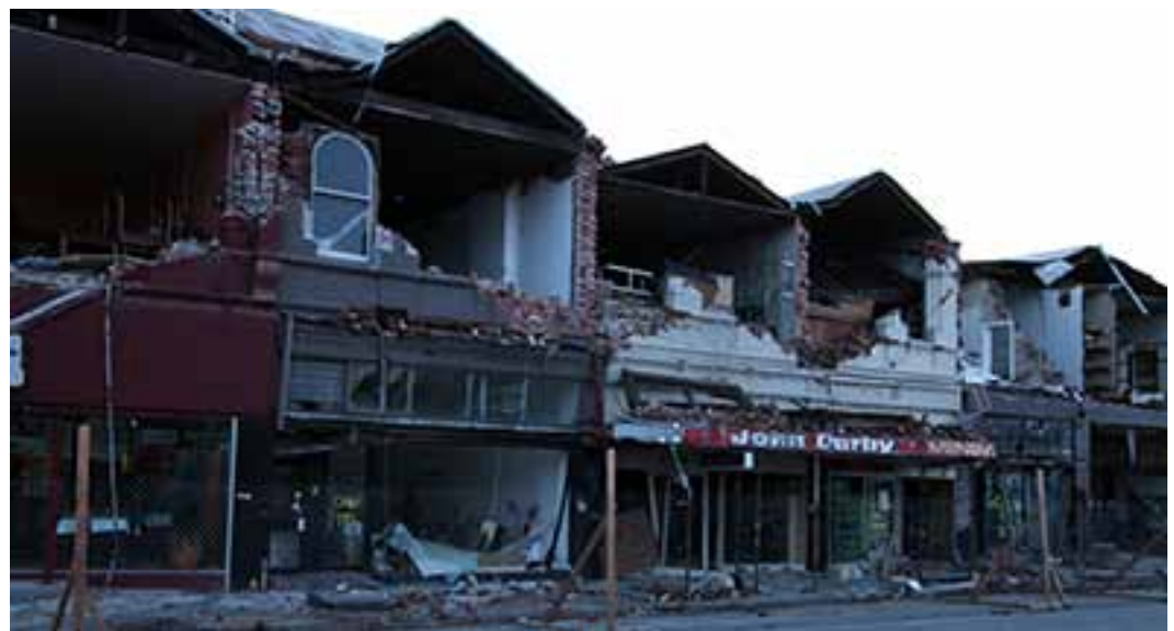
During the February earthquake two-story masonry structures suffered complete facade damage in the Christchurch historical district.
