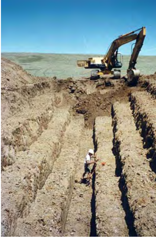
100 ft long trench, 15 ft deep, in the lower part of the Pierre Shale near Roxborough Park East, southwest of Denver, CO
