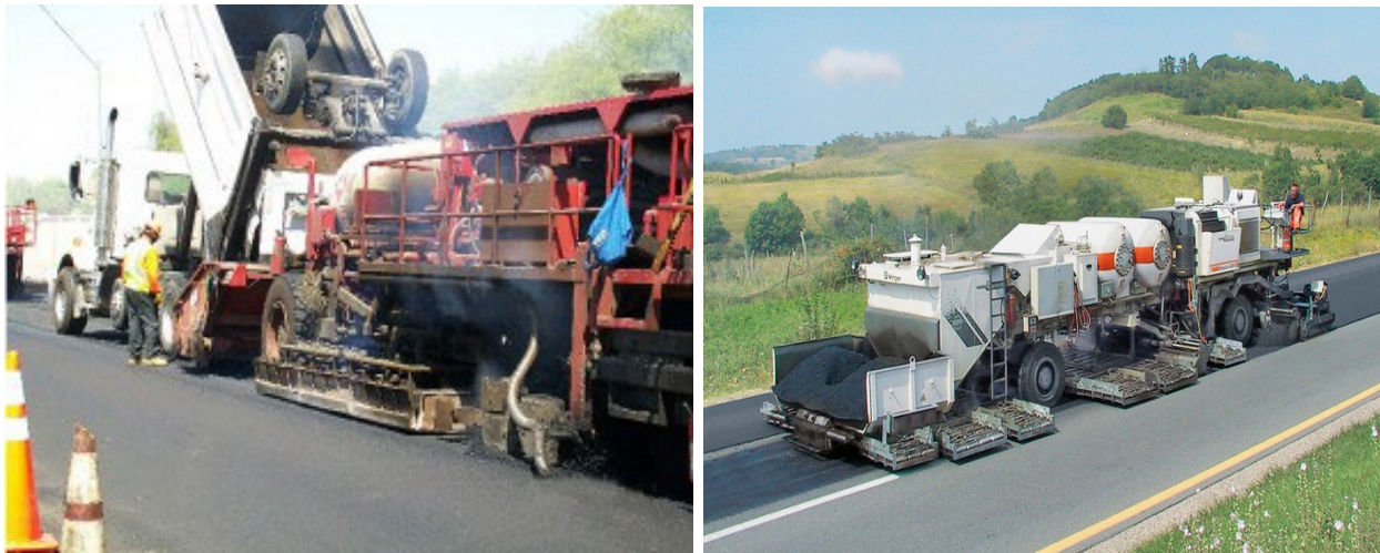
Figure 8.18 Photos of Heating and Remixing Equipment
