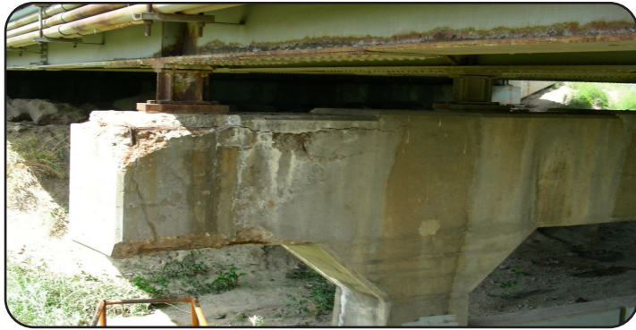
Image 26. Corrosion on US 50 ML over Fountain Creek
