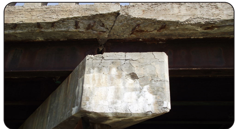
Image 14. Cracks and Deterioration on the Underside of US 6 ML over Frenchman Creek (B-27-D)
