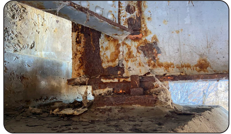
Image 12. Rusting and Deteriorating Bearing on SH 114 over Cochetopa Creek (K-09-B)
