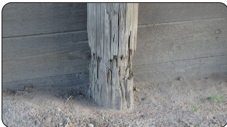
Image 13. Decay on Pile of US 385 ML over Draw (A-27-A)
