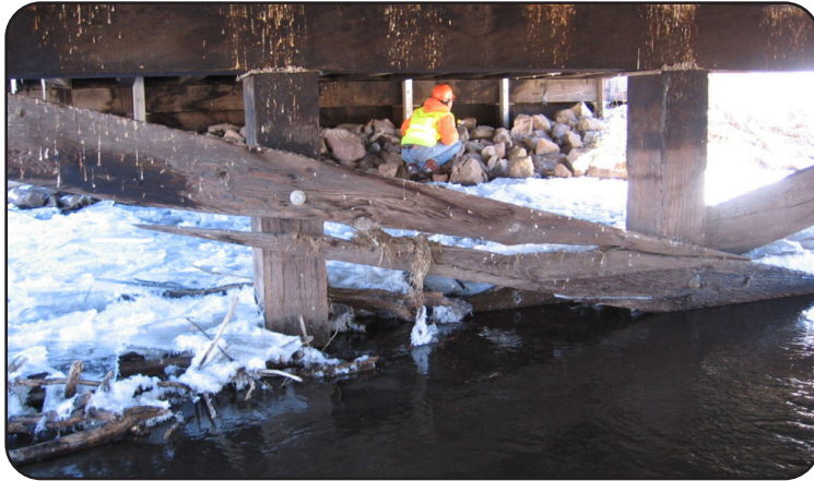
Image 11. Split Wood on Bracing on SH 114 ML over Saguache Creek (L-11-C)
