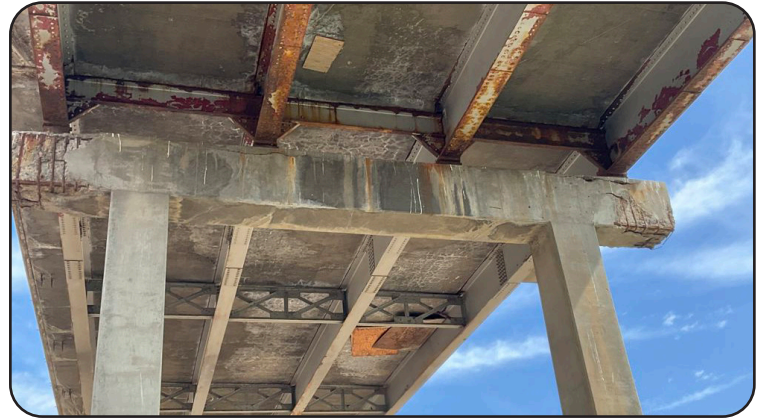
Image 9. Deteriorating Concrete and Spalling on Underside of I-25 NB over US 160, CR 10, RR Spur (N-17-AC)
