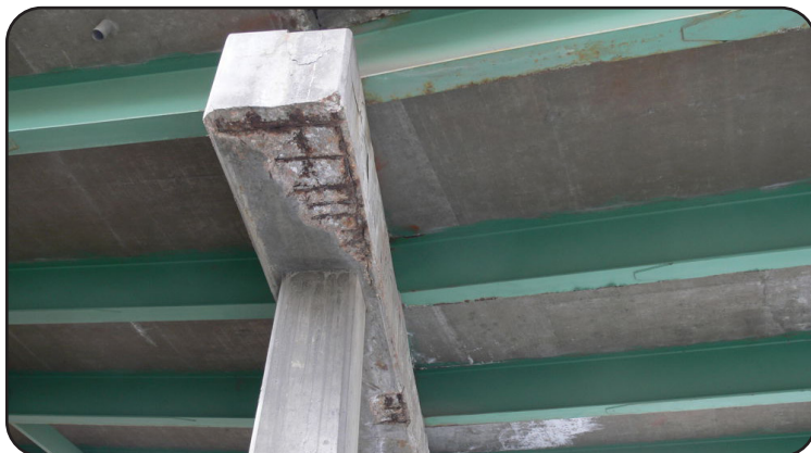
Image 10. Exposed Rebar and Spalling on I-70 WBND Ramp to US 6 over Clear Creek (F-15-BM)
