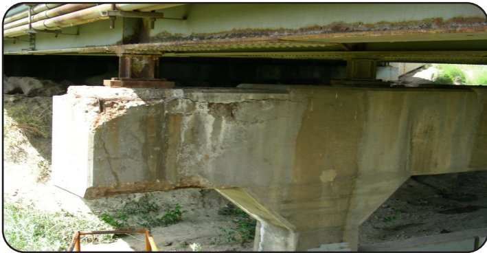
Image 29. Corrosion on US 50 ML over Fountain Creek
