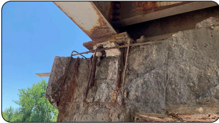
Image 8. Exposed Rebar and Deteriorating Substructure of US 85 over Fountain Creek (J-18-M)
