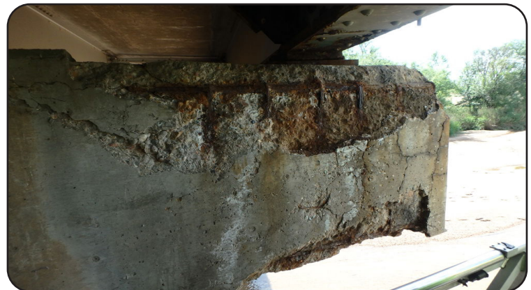
Image 11. Corroded Concrete and Exposed Rebar on US 50 ML over Fountain Creek (K-18-L)
