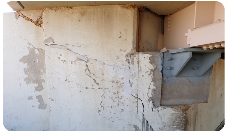
Image 11. Cracking and Deterioration on US 40 ML over Draw
