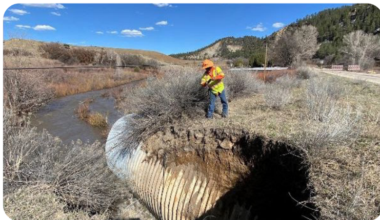
Image 11. Spring erosion on SH 151 over Stollsteimer Creek
