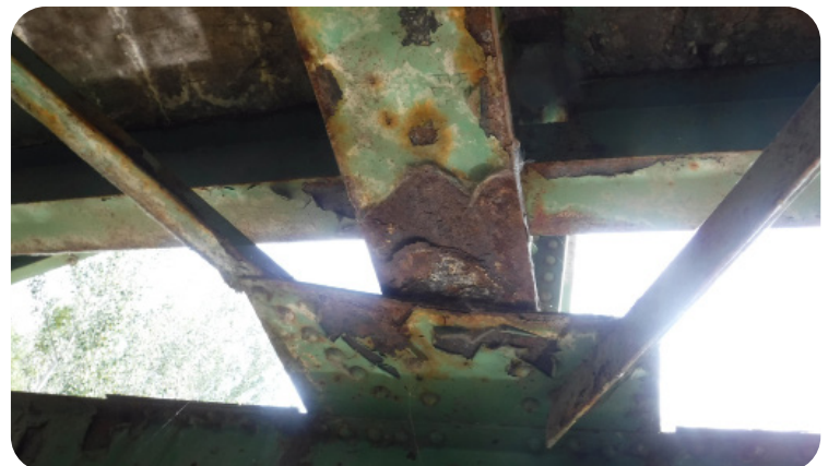
Image 7. Rust and Deterioration on US 6 over Elk Creek (F-06-A)
