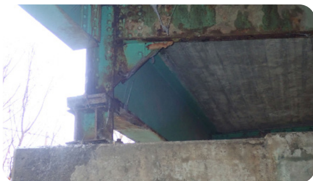
Image 10. Corroded and Rusting Bearings on US 160 ML over Florida River (P-05-B)
