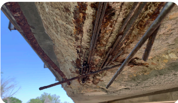
Image 9. Exposed Rebar on I-76 ML EB over US 34 Spur (C-22-BG)
