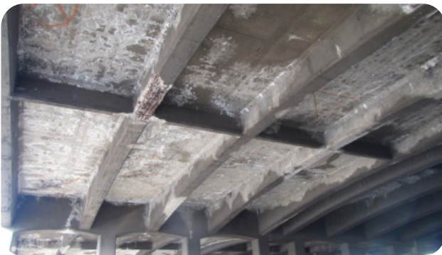
Image 8. Delamination and Exposed Rebar on US 6 ML over SH 121 ML (F-16-O)
