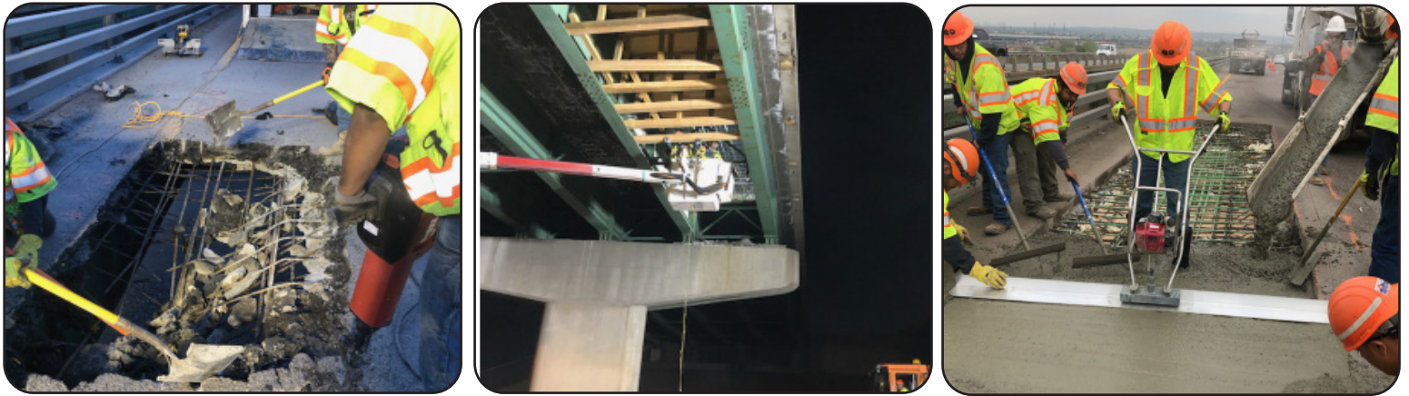
Image 21-23. Emergency Deck Repairs on I-270 ML WBND over SH 265 ML & UPRR (E-17-IH)
