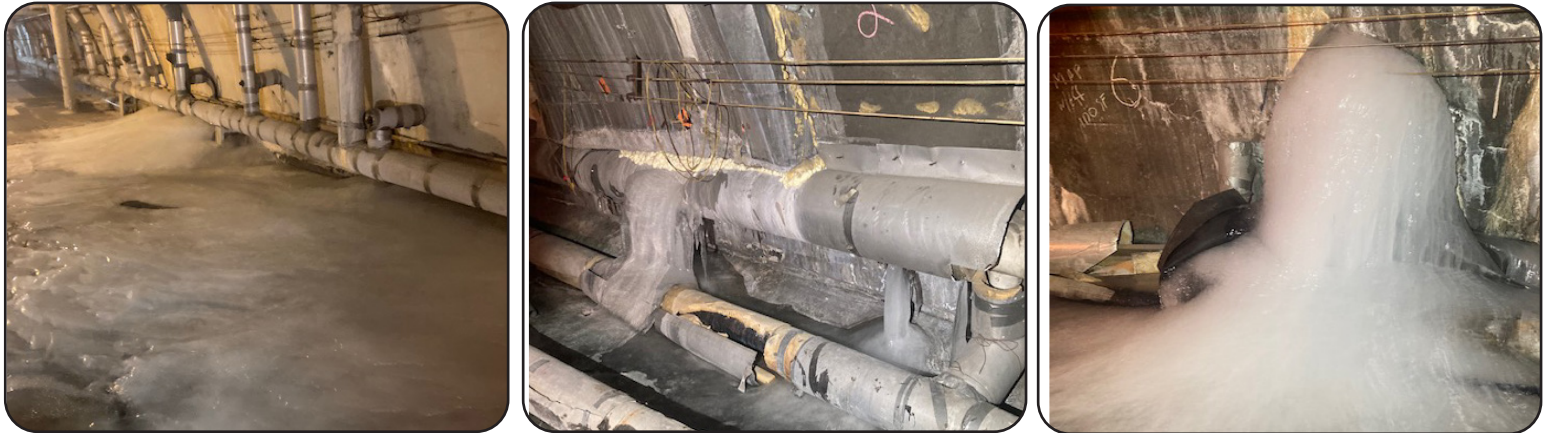
Image 1-3. Ice Caused by Water Infiltration in the Plenum Liner of Eisenhower Johnson Memorial Tunnels
