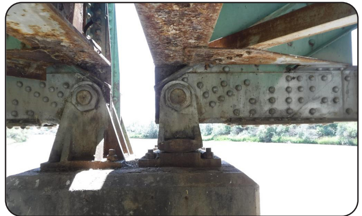
Image 10. Deterioration of Bearings on SH 92 ML over Gunnison River (I-05-V)
