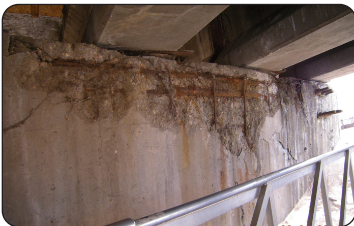
Image 12. Severe Abutment Deterioration on I-270 EBND over S. Platte River (E-17-IE)
