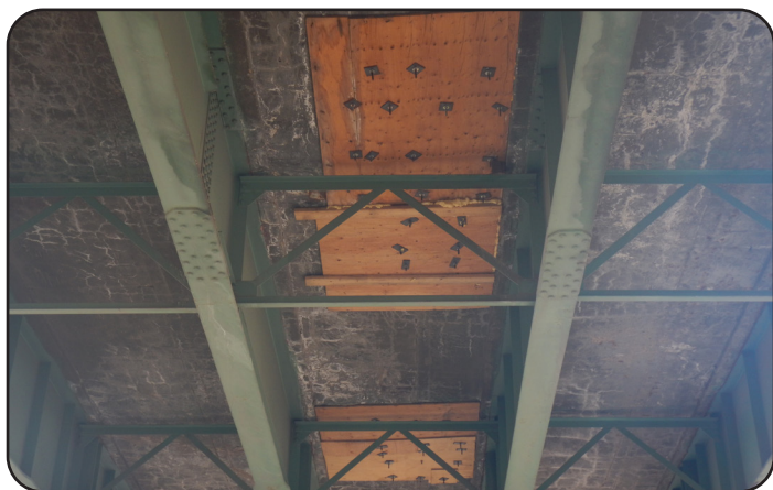
Image 11. Severe Deck Deterioration on I-270 WBND over SH265, UPRR, BNSF RR (E-17-IH)
