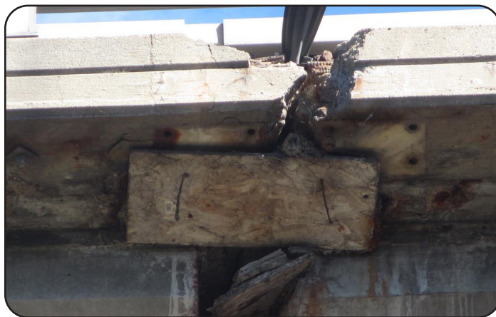
Image 10. Severe Deck Deterioration on I-270 WBND over S. Platte River (E-17-ID)
