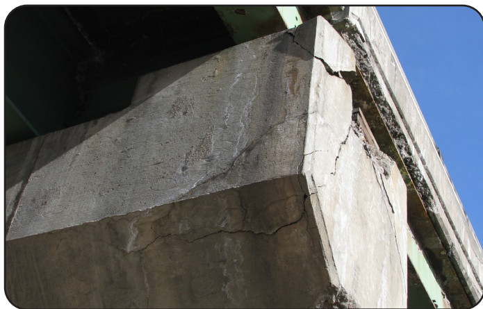
Image 9. Severe Pier Deterioration on SH 6 over Sand Creek (E-17-AT)
