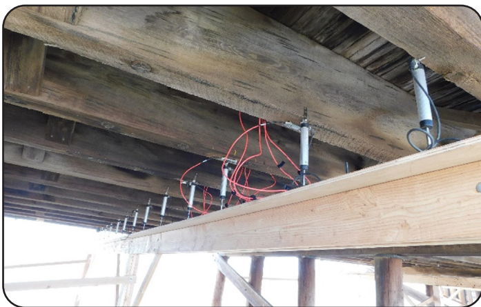
Image 11. Load Testing Sensors Measuring Displacement on US 36 over Vega Creek in Washington County
