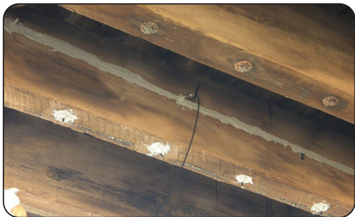
Image 12. Epoxy Injection of Existing Timber Girder Splits on US 36 over Vega Creek in Washington County
