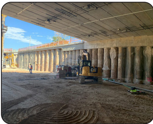
Image 14. Construction Operations at the Lowered Roadway Between York St. and Colorado Blvd.
