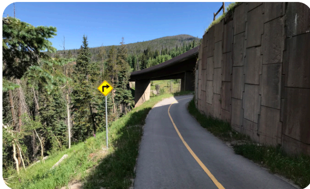
Image 7. Substandard Curve Geometry at I-70 over Polk Creek Viewed from Recreational Path
