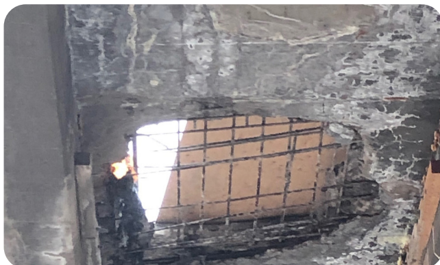
Image 3. Hole In Deck of I-76 over York St Viewed from the Underside
