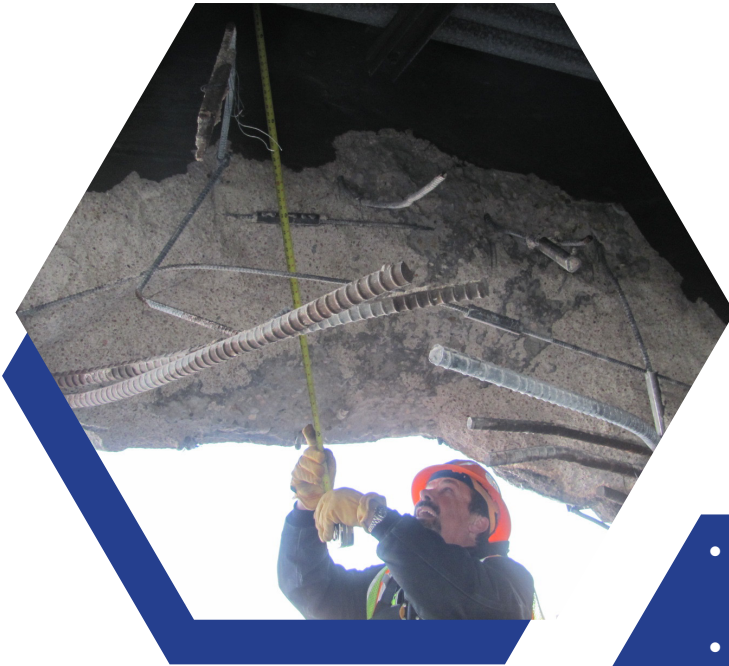
Image 15. Impact Damage from Truck Strike Speer Blvd over I-25 in Denver (E-16-EW)
