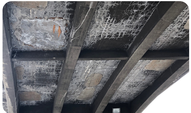
Image 2. Deteriorated Deck Underside on I-76 over York St
