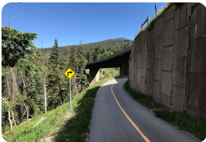
Image 5. Substandard Curve Geometry at I-70 over Polk Creek as Viewed from the Recreational Path
