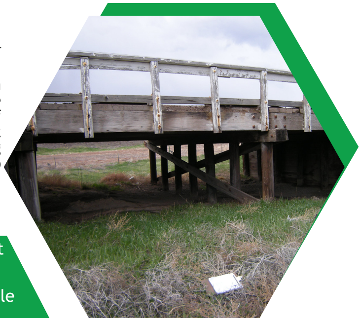
Image 13. Deterioration of I-70 Service Rd over Draw (F-20-L)
