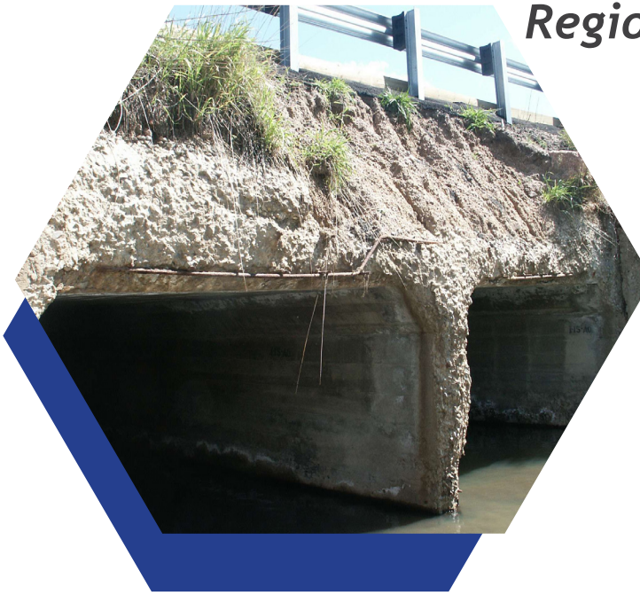
Image 12. Deterioration of Concrete on US 24 over Draw in Teller County (I-15-AO)
