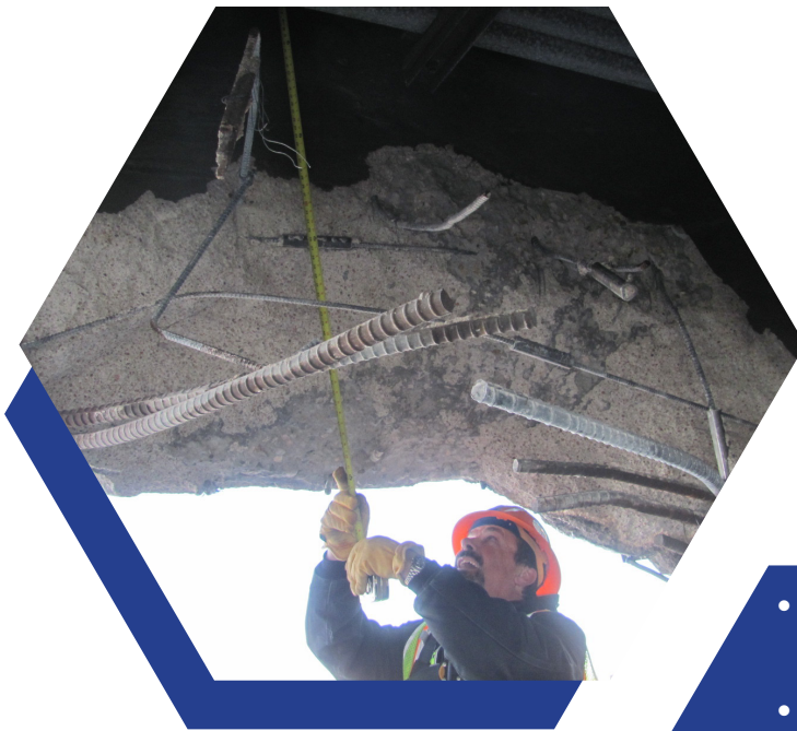
Image 15. Impact Damage from Truck Strike Speer Blvd over I-25 in Denver (E-16-EW)
