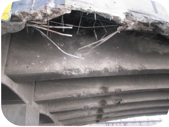
Image 7: Impact Damage to Speer Blvd Northbound over I-25 (E-16-EW)
