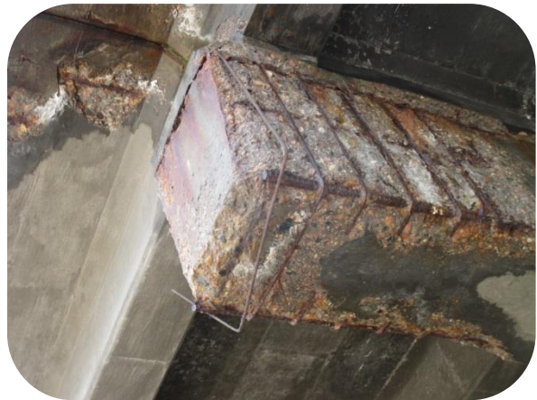
Image 8. H-17-CI Pier Cap Deterioration
