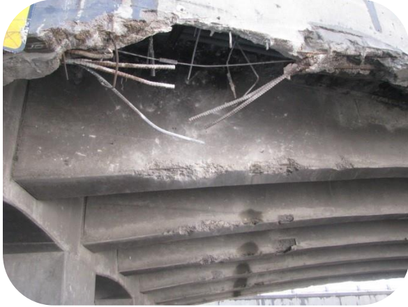
Image 9: Impact Damage to Speer Blvd Northbound over I-25 (E-16-EW)
