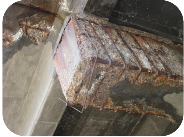
Image 9. H-17-CI Pier Cap Deterioration
