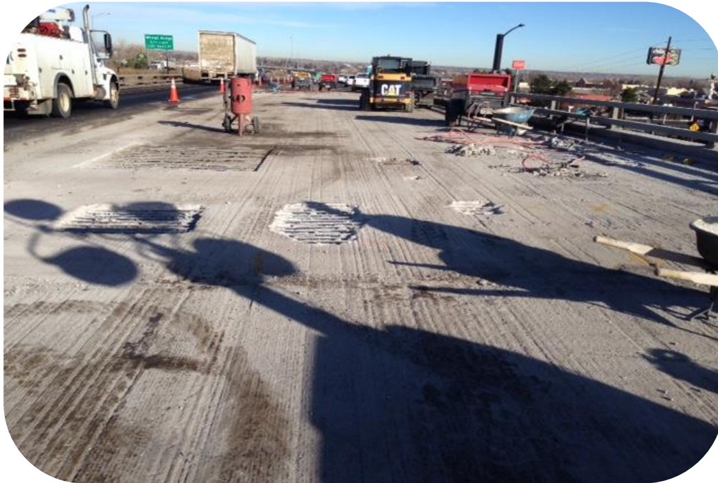
Image 7. Multi-lane Closure on I-70 over West 32 nd Ave (E-16-HF) for Bridge Deck Repairs
