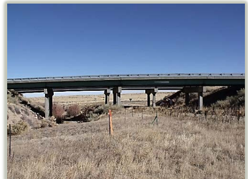
Image 4. Existing I-25 SB over CO RD 640 and Butte Creek and I-25 NB over CO 103 and Butte Creek (N-17-BN/S)
