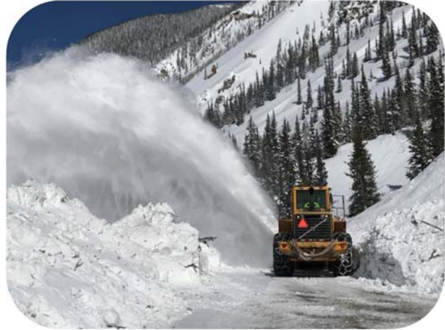
CDOT Maintenance crews perform avalanche mitigation on Red Mountain Pass in southwest Colorado. CDOT’s snow and ice control program ensures safe travel for Colorado’s citizens during inclement weather.
