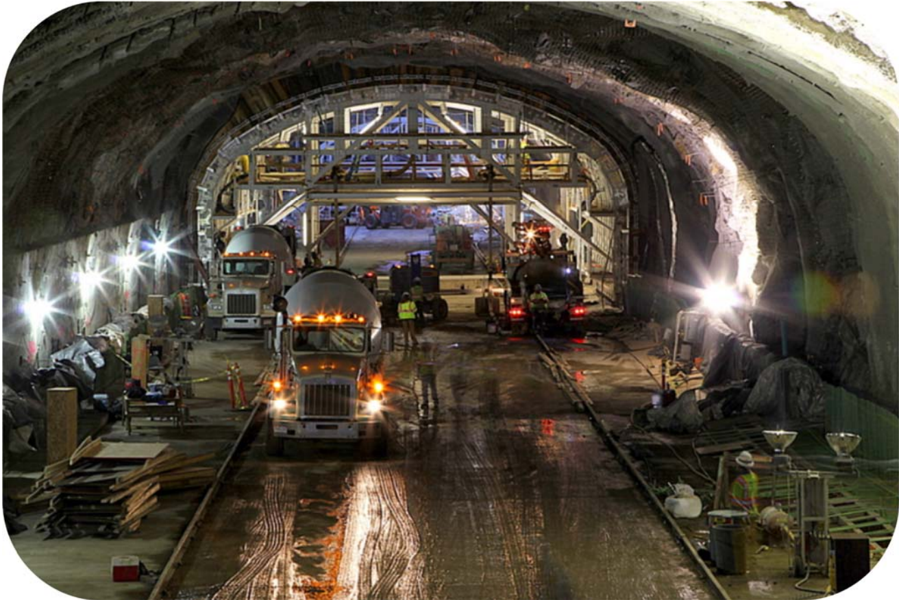
Reconstruction of the Veterans' Memorial Tunnels, along I-70 near Idaho Springs, in 2014.
