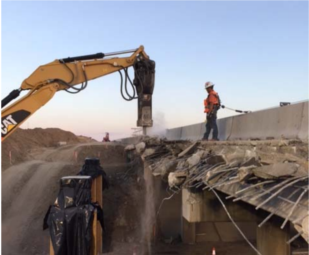
Demolition in progress for a CDOT project that added a climbing lane on southbound Interstate 25, south of Berthoud.
