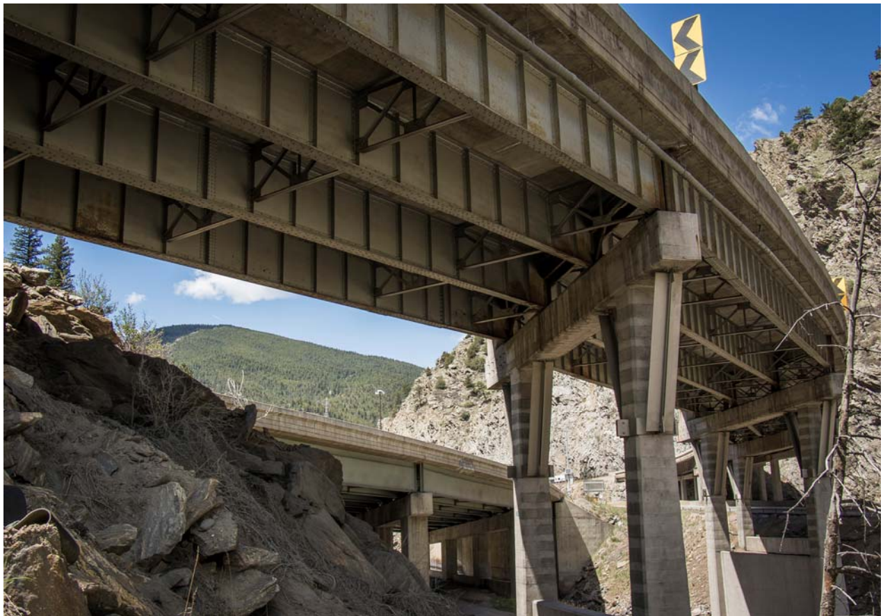
CDOT maintains more than 3,400 vehicular bridges, including this bridge on Interstate 70, east of Idaho Springs.
