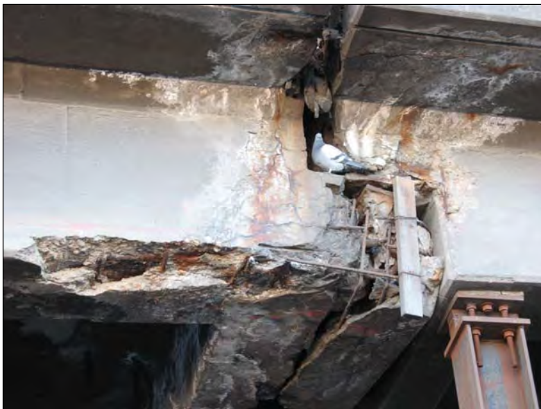
Joint damage on the Interstate 70 viaduct east of downtown Denver. About $60 million per year for financing the viaduct's replacement is included in the cost estimates on the following two pages.
