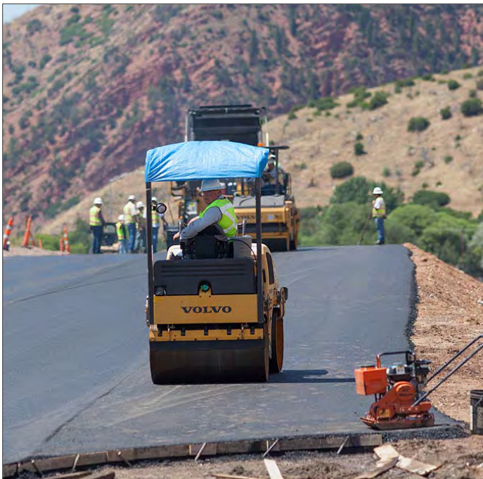
A CDOT contractor places new asphalt pavement and compacts it to specified densities as part of the Grand Avenue Bridge project in Glenwood Springs.
