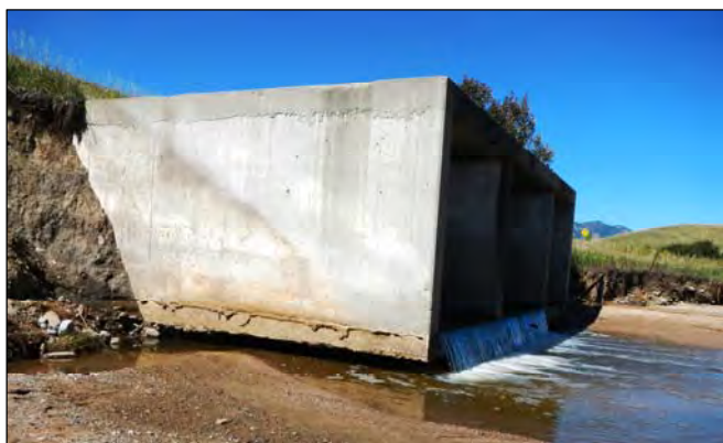
Vehicles on State Highway 128, southeast of Boulder, regularly travel over this concrete box culvert, which faces scour concerns. At the culvert outlet, water has eroded three feet from the bank of Coal Creek.
