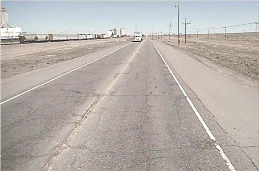
This stretch of pavement, on State Highway 2C at the northwest boundary of Rocky Mountain Arsenal National Wildlife Refuge, has a Drivability Life of zero years. Extensive surface cracking is one factor placing the pavement in the Low Drivability Life category.
