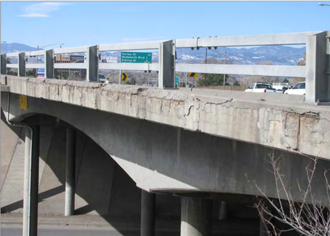
A deteriorating overhang on a bridge on Interstate 70, near Lakeside Amusement Park in Denver. CDOT maintains this bridge that was built in 1966, ensuring that concrete does not fall on vehicles traveling underneath.
