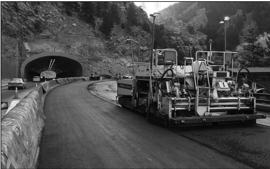
An asphalt paver places fresh, uncompacted asphalt pavement near the Twin Tunnels east of Idaho Springs.
