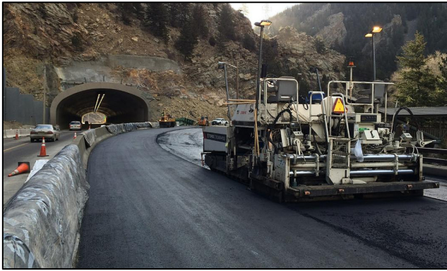
An asphalt paver places fresh, uncompacted asphalt pavement near the Twin Tunnels east of Idaho Springs.
