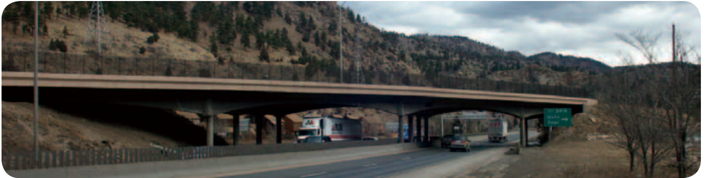
Added to the poor list, I-70 Business Route over I-70, Idaho Springs (Structure number F-14-Y)
