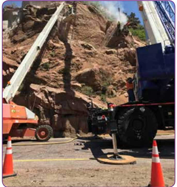
Rock bolt installation on US 24 Ute Pass just west of Manitou Springs was part of the corridor mitigation project.
