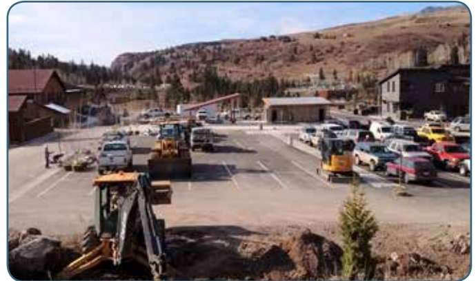
The new 110-space San Miguel County park and ride, located on Lawson Hill off CO 145, between Telluride and Mountain Village.
