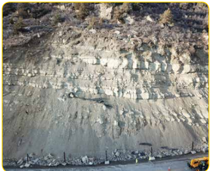
Crews remove a failed anchor mesh section on CO 133 near Paonia Reservoir.
