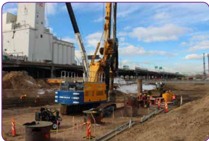
The Central 70 project will help relieve congestion and improve travel times when it is completed.
