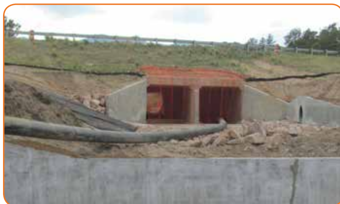
Concrete box culverts under I-25, at Monument Creek Branch, were repaired following flooding that left the structures significantly scoured.
