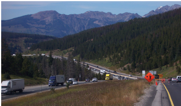
CDOT completed major resurfacing and safety improvements on I-70 west over Vail Pass. [REGION 3]
