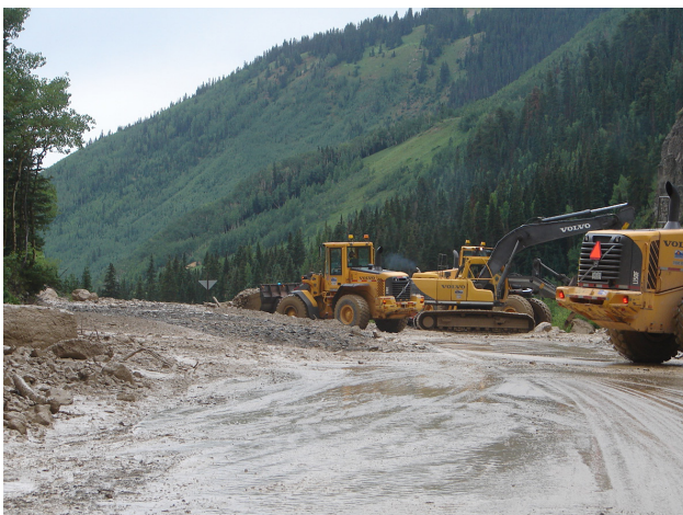
CDOT maintenance crews handle challenges brought on by Colorado's extreme weather, including mudslides like this one after an August rainstorm on US 550 north of Silverton. [REGION 5].
