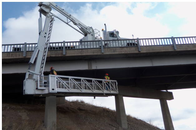
Maintenance workers conduct a routine bridge inspection on US 85 near Nunn. [REGION 4]
